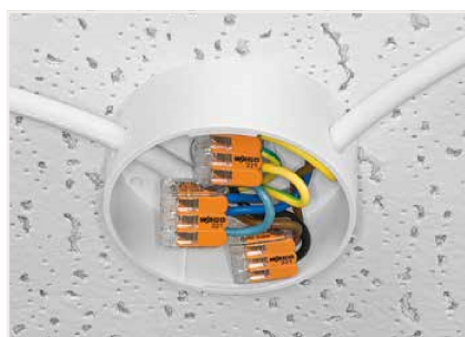
Lighting distribution in ceiling canopy
